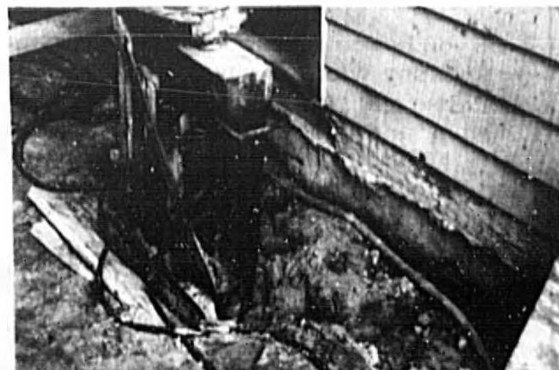
This is the only exterior indication that a Hidden Village condo near Lake Mary is sinking. The ground beneath the building settled, exposing the ragged concrete slab underneath.
