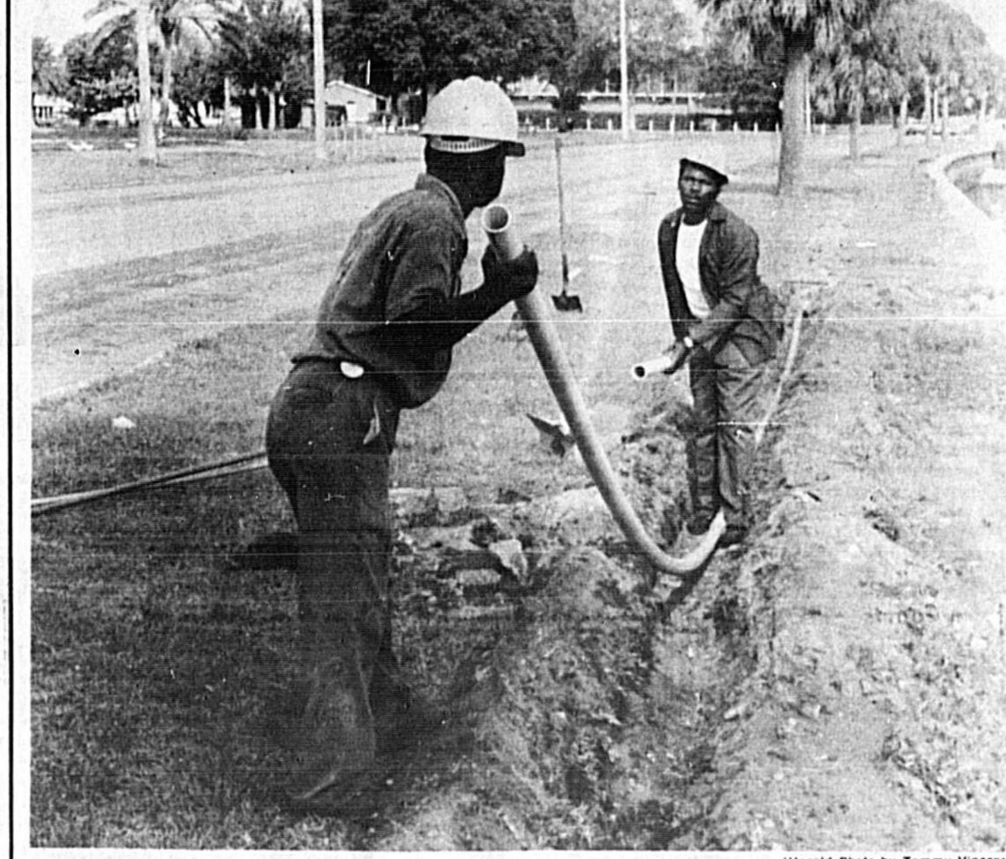
LAYING THE PIPES Sanford Parks Department employees Frank Williams and Clondike Abbott lay pipes for a sprinkler system which will water new flower beds provided by Community Improvement Project.
