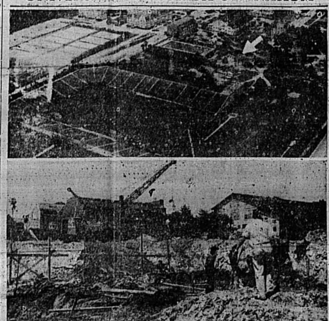
"THE UNIVERSITY OF FLORIDA'S GYMNASIUM" is fast becoming a reality as construction continues at a rapid pace. Top aerial view shows general area where gymnasium will be located (arrow) while bottom picture shows construction in progress. When completed the gymnasium will be one of the most modern plants of its kind and will house offices and classrooms of the College of Physical Education, Health and Athletics, as well as provide complete recreational and training facilities for the student body.
