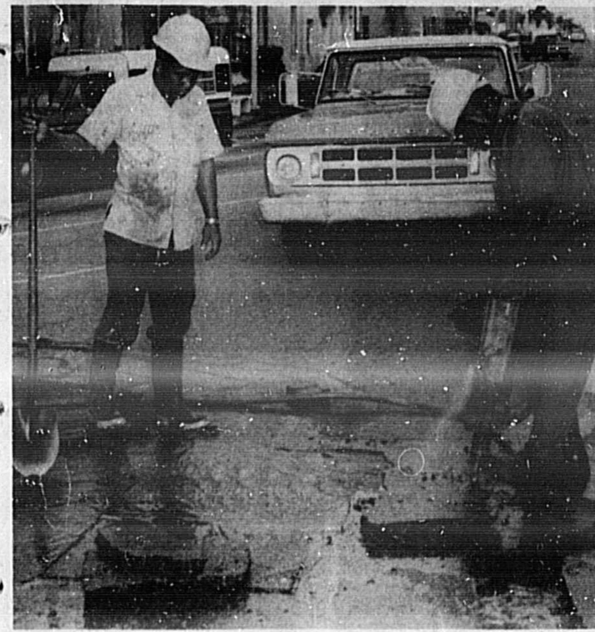
Water line break repaired. City workers were busy today repairing a service line adjacent to a water main on First Street.
