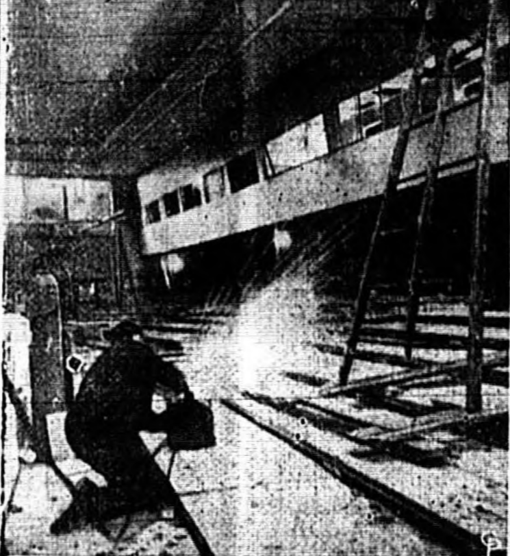
HUNTER COLLEGA in the Bronx, N. Y., is having a major operation in preparation for its occupancy by the United Nations Organization's Security Council. Here a welder is making the sparks fly in the convention room, formerly the college's main gymnasium. Note the layout in the background where seats will fan out. The upper center balcony is where the members of the press will sit. (International)
