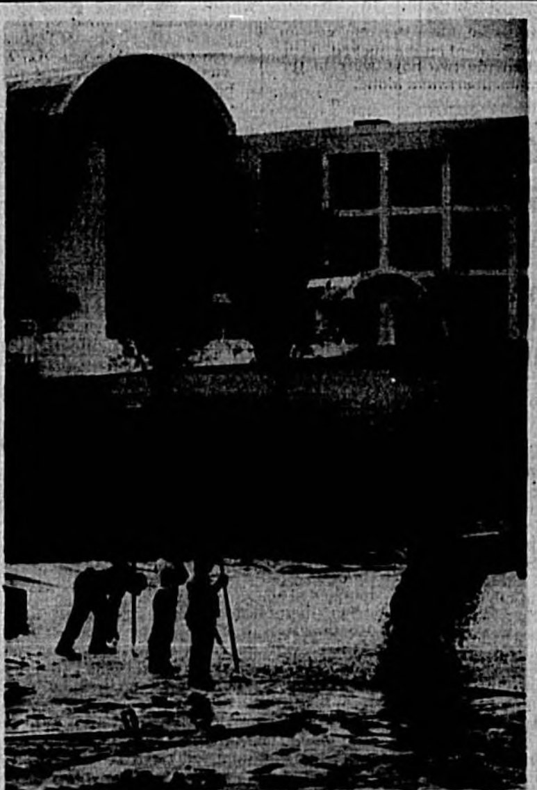
Pulling the plug Workers from Environmental Care Inc. drained the fountain in front of American Automobile Association's national headquarters in Heathrow yesterday. The workers drained the pond to reinforce its bottom with gravel.
