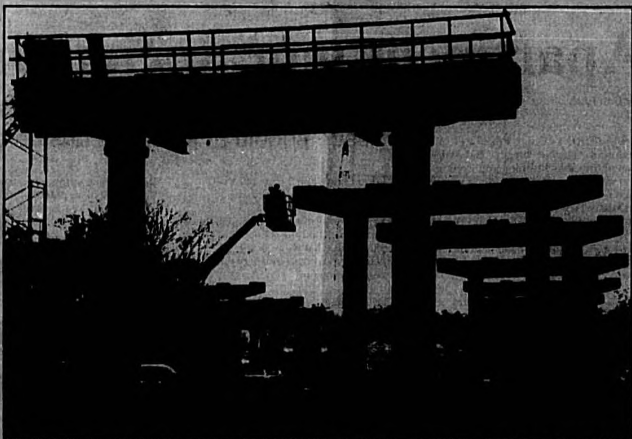
The supports go up for the roadway that will cross over Old Lake Mary Road and the railroad tracks near the Airport Boulevard intersection. Construction work continues on the GreenWay (417) extension to that will connect the toll road with I-4.
