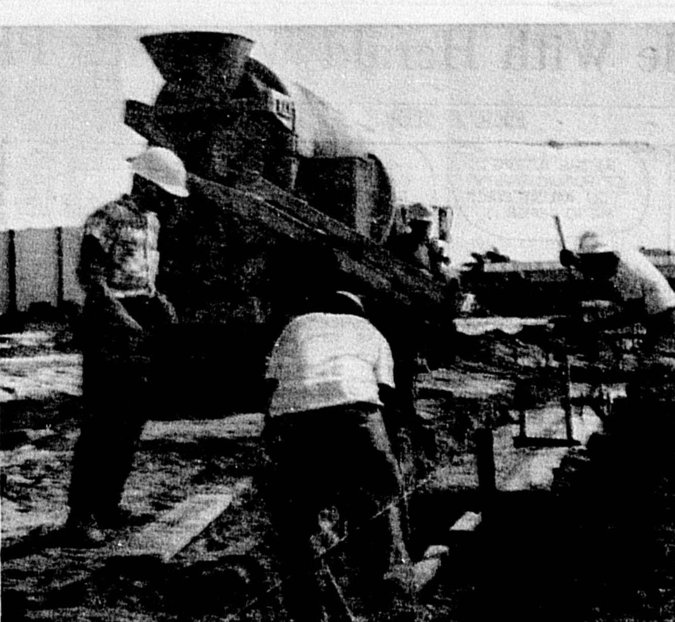
WORK IS progressing on the new Montgomery Ward complex in Seminole Plaza at Casselberry. Footers have been poured (totalling 1,003 feet in the main building alone) and the rain has been beneficial in packing down the fill dirt. Fred Snow, project manager for Sutler Construction Corporation, has set a February completion date. If all goes according to schedule, steel work will start Oct. 6 and block laying around Oct. 20.
