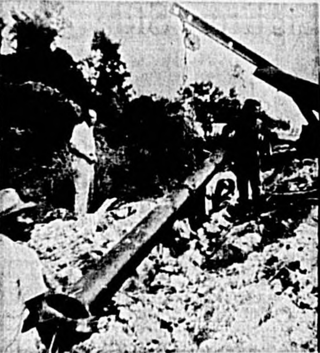
EIGHT INCH water lines are being installed by Casseberry Utilities from the Queen's Mirror South plant to give increased pressure for many homes in the area. Work is expected to be completed by the end of the week. (Herald Photo)
