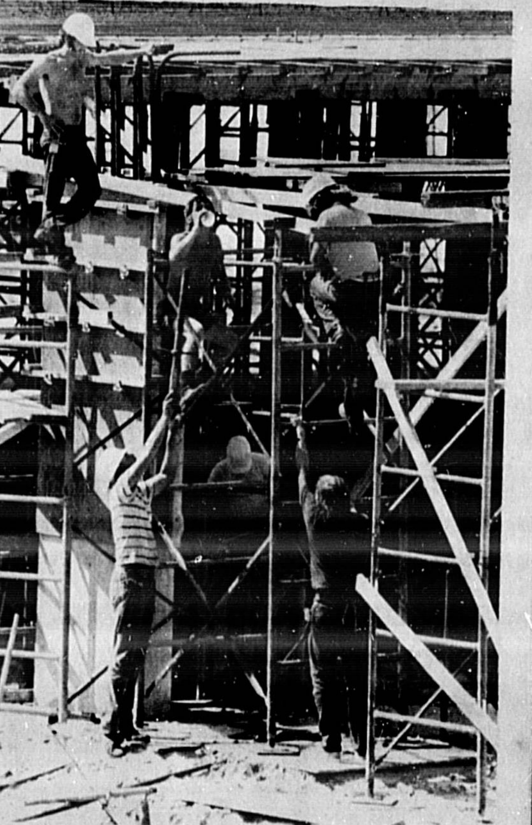
IT'S MY TURN NEXT! CONSTRUCTION WORKERS take an ice water break on the scaffolds in the afternoon heat at Seminole Junior College at Sanford. Forecasts call for temperatures to continue in the 90s for the next couple days and cold ice water will be in demand.
