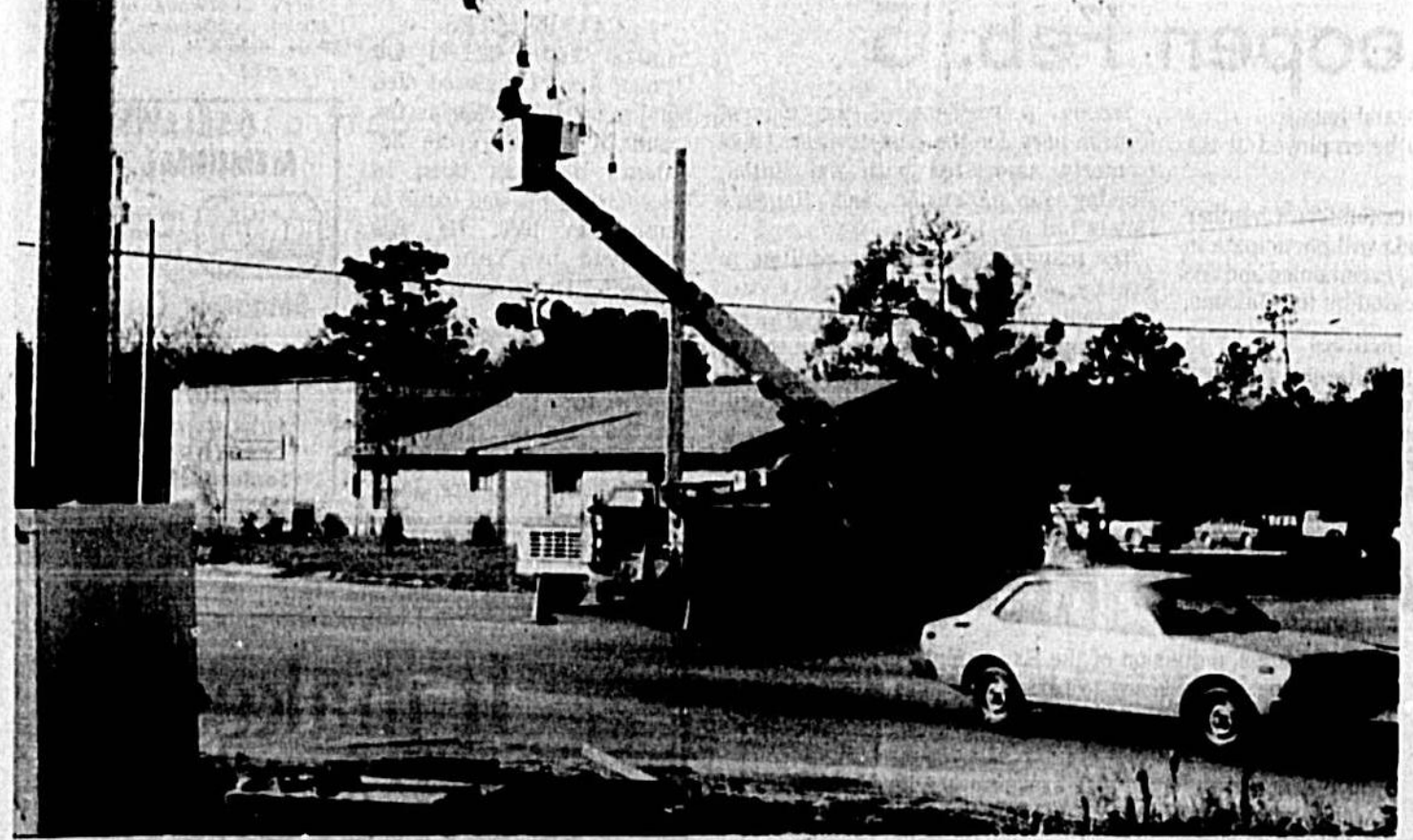
Traffic lights at 24th Street and Airport Boulevard, being installed for Seminole County by Control Specialist of Orlando, are expected to be operating Tuesday on a fixed timing basis. They replace a blinker at the intersection, which has been the scene of many accidents and traffic problems. The controls will include a protected left turn signal.
