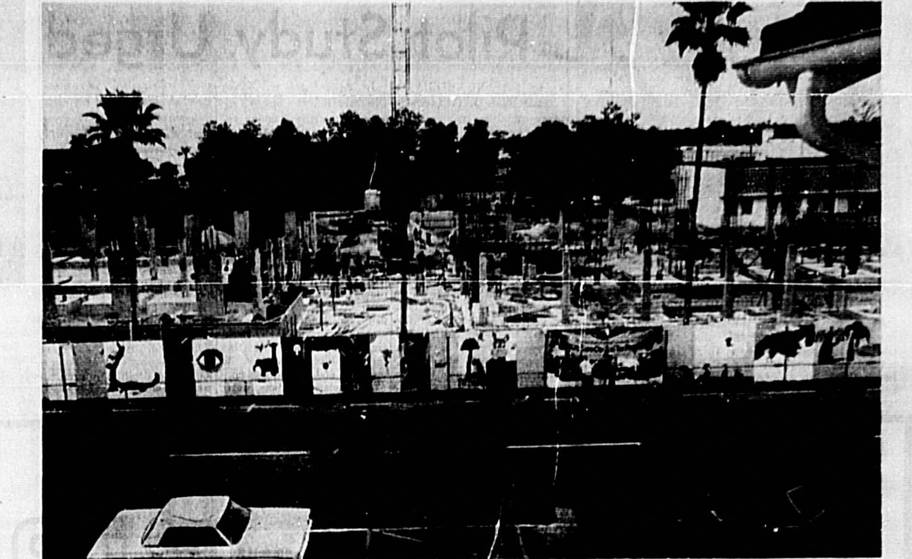
ON THE OTHER SIDE OF THE 'ZOO CURTAIN' WORK CONTINUES on the Seminole County Court House, located on Park Avenue in Sanford. The $4.2 million structure is scheduled for completion April 1972. Herald Staffer Bill Vincent took this shot from the top floor of the Sanford City Hall, located directly across the street from the present construction site.
