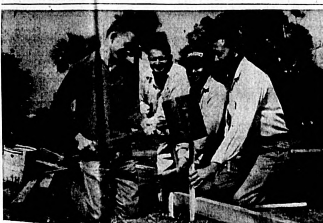
ALL IN A DAYS WORK! But this is mighty happy work as the Seminole High School Physical Education Court got underway Saturday. Laying out the "latter boards" are (left to right) Tommy Hittel, Phil Westgate, Jeff Willmon, and Claude Hittel. The project is sponsored by the Seminole High School P-T-A. (Photo by Bergstrom)
