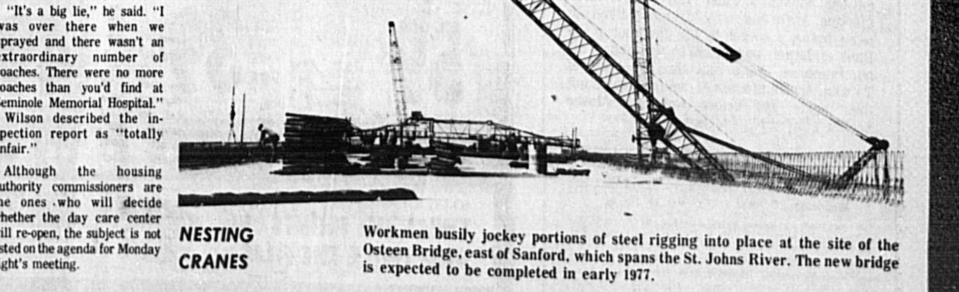
Workmen busily jockey portions of steel rigging into place at the site of the Osteen Bridge, east of Sanford, which spans the St. Johns River. The new bridge is expected to be completed in early 1977.
