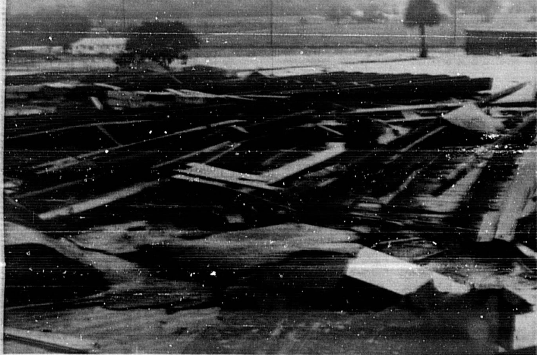
ICE PLANT of City Products at Rand's Yard lost most of its roof to Wednesday's storm. Herald photographer Bill Vincent Jr. climbed a 100-foot ladder to snap this picture of the torn-up roof.
