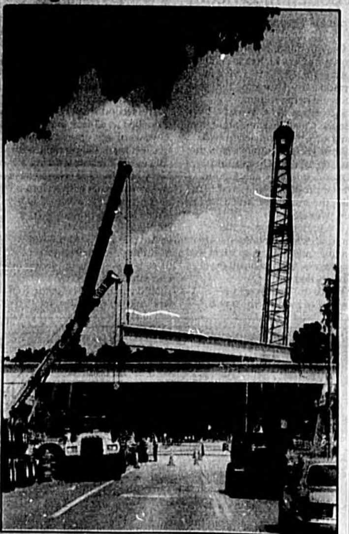
Workers place bridge supporters over Upeala Road in Sanford as part of the GreeneWay expansion project. Herald photo by Tommy Vincent
