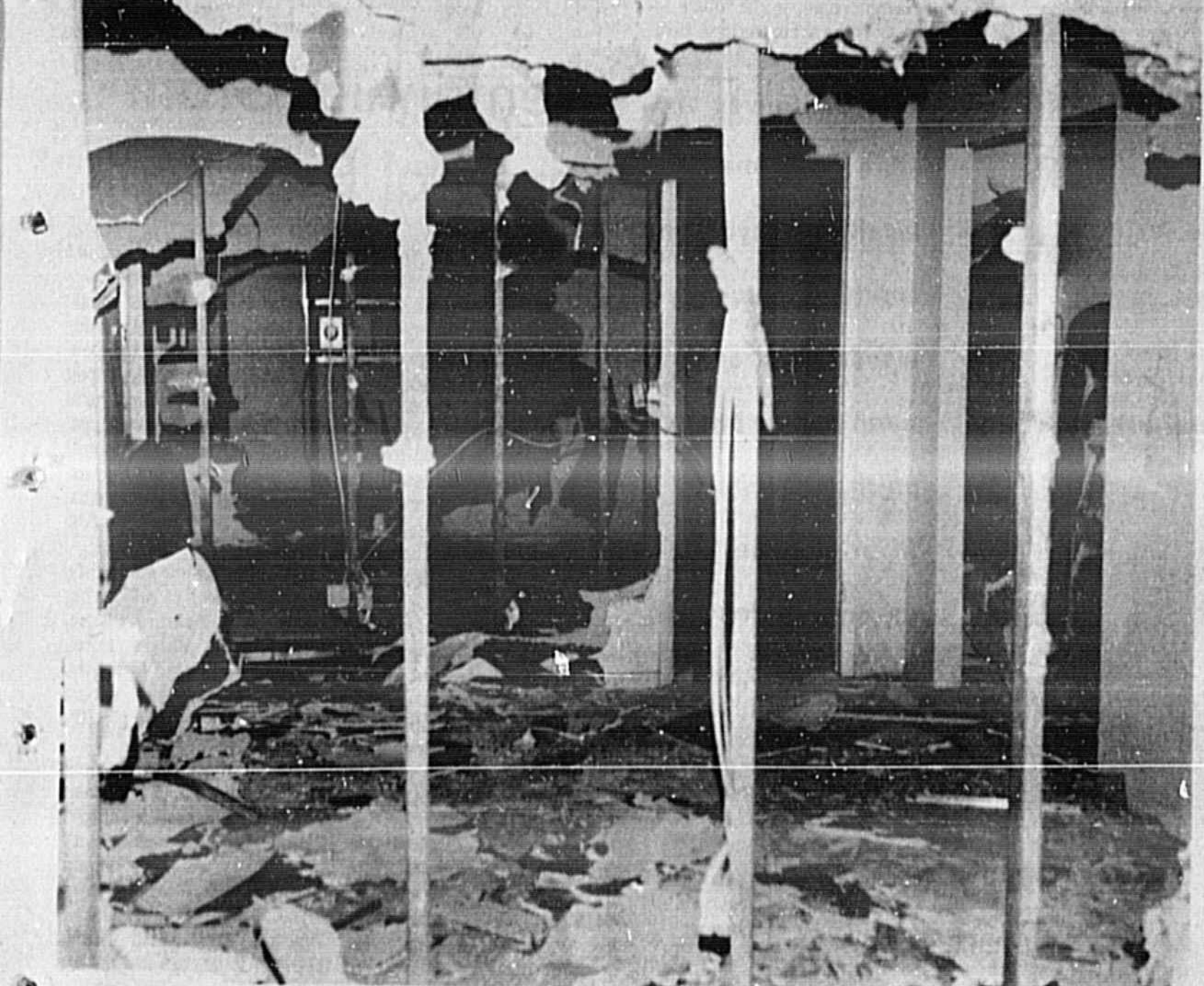
VANDALS RUIN LOCAL HOUSES Three houses under construction in Academy Manor subdivision in Sanford were hit by vandals Tuesday causing approximately $20,000 in damage to the three buildings. Sanford patrolman Joe Dillard said an electric range was completely destroyed, windows were torn out from the walls, and inside room separators were knocked down. Most severely damaged house is located at 223 Yale Avenue with estimates of the damage totaling $10,000. The houses are owned by Kingswood Estates of Casselberry. Sanford police are continuing the investigation.
