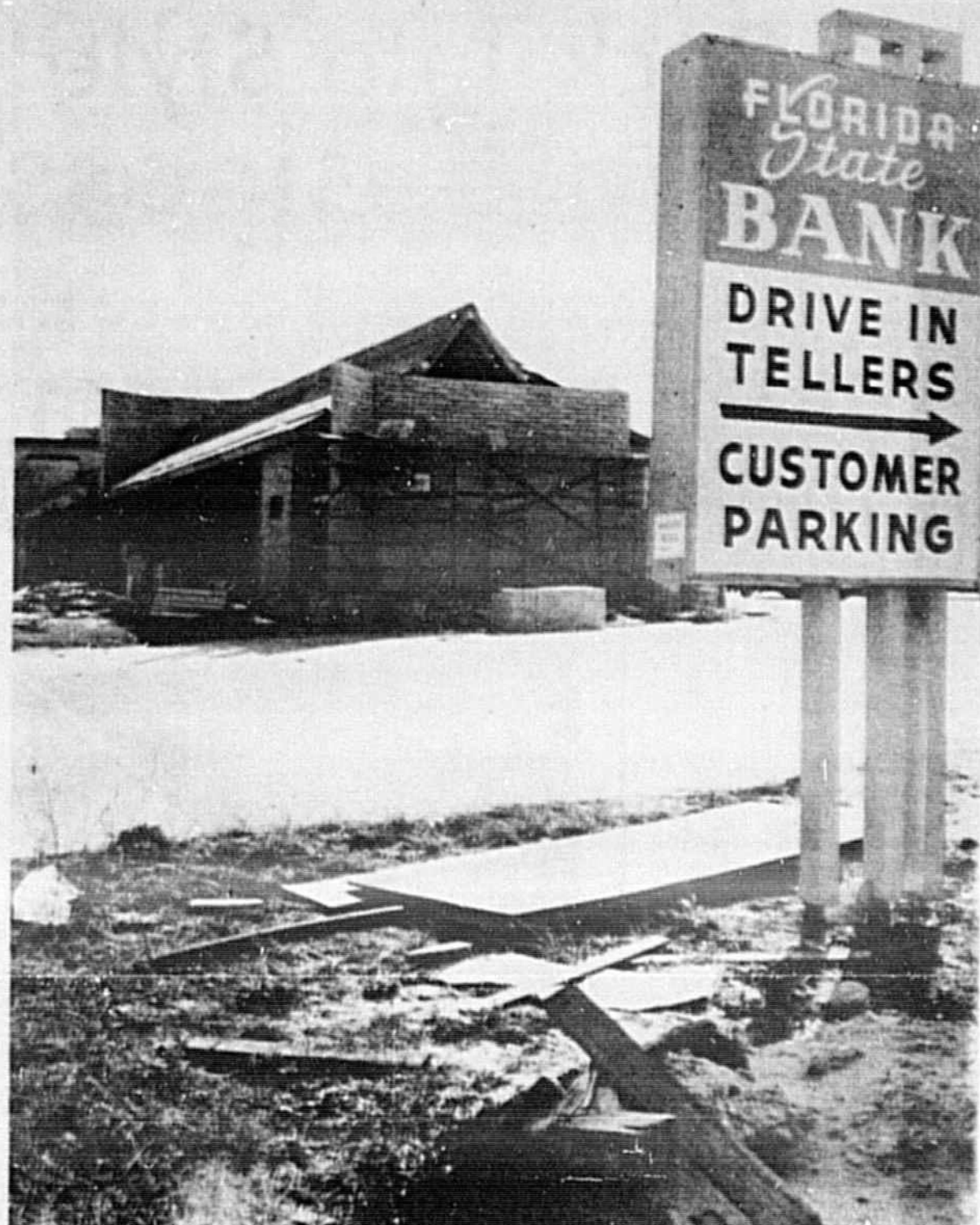
FLORIDA STATE Bank officials say construction of four new "speed lane" drive-in teller windows at the Sanford facility is expected to be completed in March...
