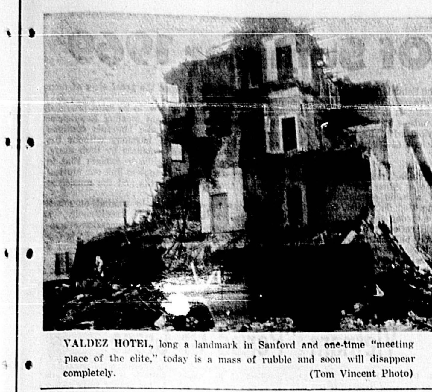
VALDEZ HOTEL, long a landmark in Sanford and one-time "meeting place of the elite," today is a mass of rubble and soon will disappear completely. (Tom Vincent Photo)
