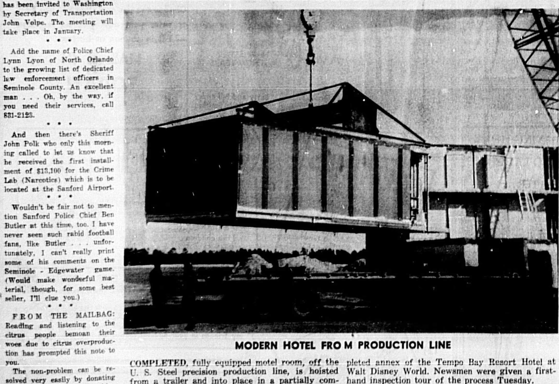
COMPLETED, fully equipped motel room, off the planned annex of the Templo Bay Resort Hotel at U. S. Steel precision production line, is hoisted Walt Disney World. Newmann were given a first-hand inspection tour of the process Tuesday.
