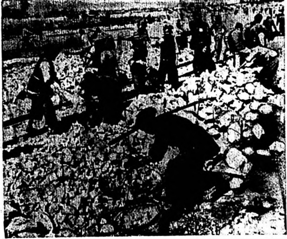
IN THE INNERMOST REGIONS OF FREE CHINA, women of the north have helped to build a railroad by hand. In the picture above, they grade and prepare the site for a track. Each stone is carried by shoulder yoke salvaged from railroads in Japanese territory. (International)
