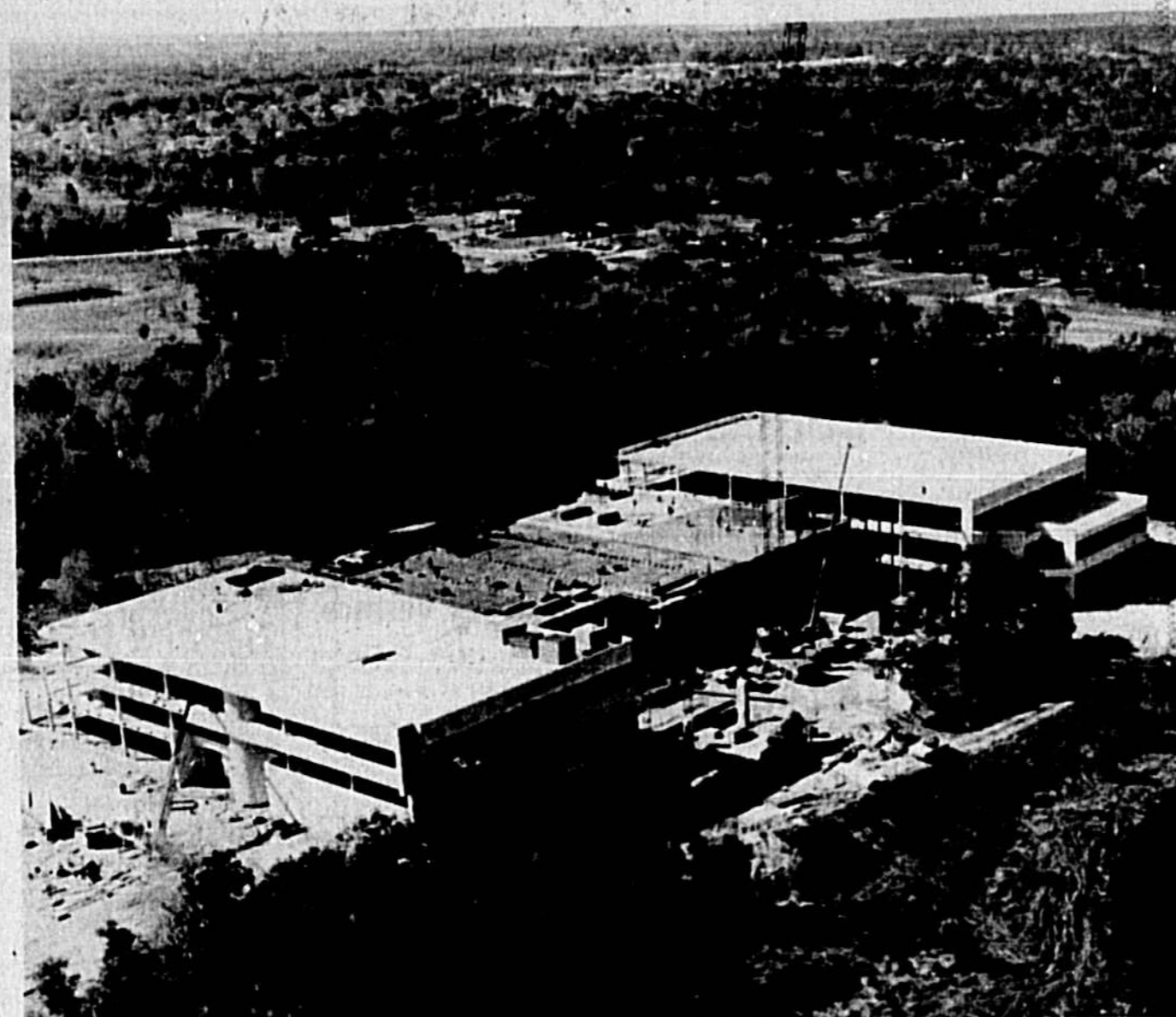
United Telephone Systems-Florida Group's new headquarters as seen in aerial photo taken about a month ago.
