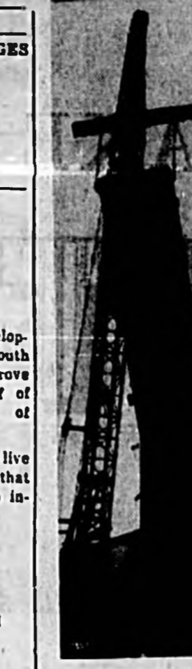
A CRANE LIFTS A 56-foot tank into position in San Jose, Calif., as an experimental boiling-water type atomic reactor nears completion. Nuclear fuel bundles will be tested under 40 feet of water within the tank to devise refueling procedures for the nuclear power station to be built in Chicago by the General Electric Company. (International)
