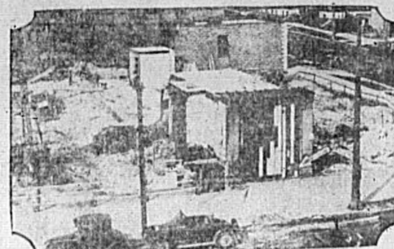
Building of the new twenty-six-story tower of the Milwaukee Gas Company is a problem. Lincoln Hotel was one of the buildings razed, but the rooms could not be wrecked until the padlock device had expired. Workers decided to erect the building around them.
