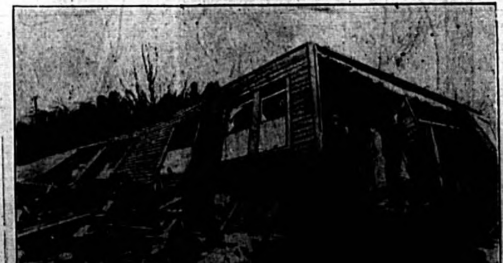
Two persons lost their lives in this wreckage of their home which was demolished by a tornado in the vicinity of Pyrite, Ala. The victims, Glenn Parham and his wife, were among 17 killed by similar disturbances about the same time in sections of Alabama, Georgia and Florida. (Associated Press Photos)
