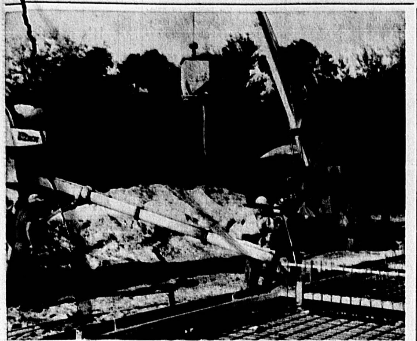
LATEST PHASE in the Casselberry Utilities' expansion program at the sewage treatment plant is under construction. A $14,000 building permit has been issued by the city for a 200,000 gallon aeration settling tank that will provide for service to an additional 600 homes. Due to the size of the project, the crane is employed to pour concrete in the center of the large tank. (Herald Photo)
