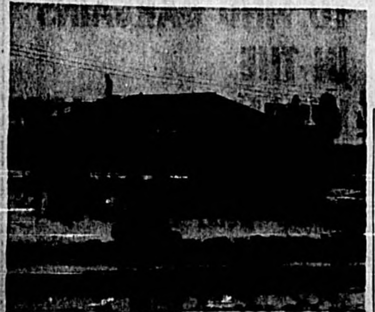
PRESENTLY HALF ERRECTED is this Butler type building located east of Building Two at Sanford Naval Air Station. The building of this type are presently under construction at the SNAS. The work on this building is being done by the Carroll Daniel Construction Company, of Gainesville, Ga. (Official Photo, U. S. Navy)
