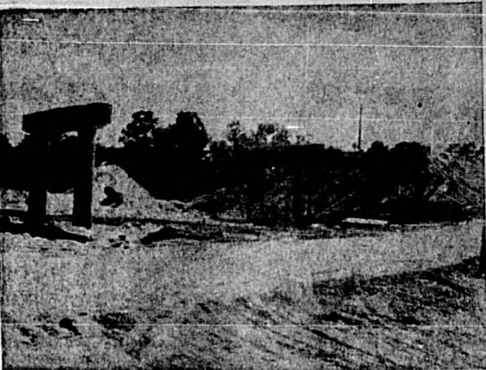
INTERSTATE 4 construction through Seminole County is progressing more rapidly than the public realizes. This top photo shows bridge piers for the cross-over at Highway 46A . . . .
