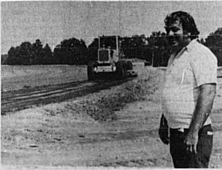
Jimmy Wilkerson watches as the track of his $750,000 JW Training Center is under construction near Oviedo. Harness race horses will be training at the facility in the winter months.
