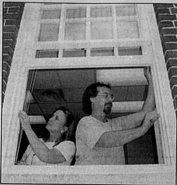
Herald photo by Tommy Vincent Chris and Leslie Stevens work on restoring a window at the old post office on First Street.
