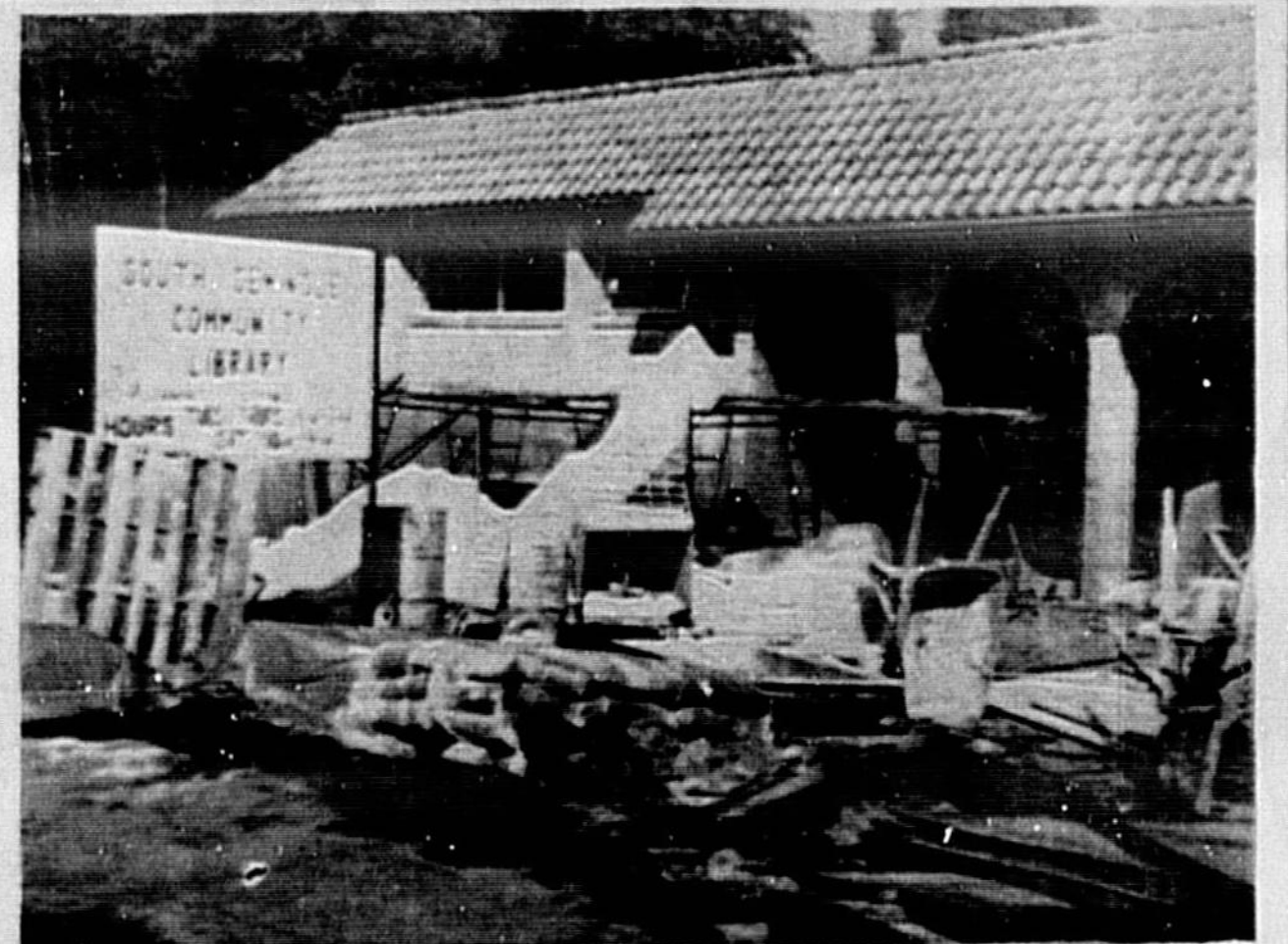
ATTRACTIVE Mediterranean style library being built by South Seminole Community Library in Altamonte Springs hides the old building. Business is being carried on there as usual. (Ray Knight Photo)
