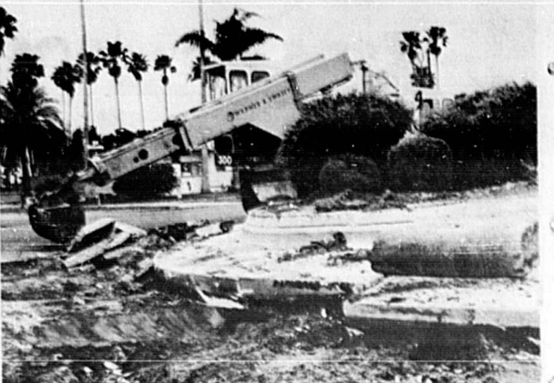
SANFORD CITY crews today began demolishing the base of the Memorial Park (handshell pier) monument and flagpole in the first phase of a $17,500 (facilitating) renovation into an attractive lakefront park. City parks director Jim Jenkins said the flagpole base will be changed from its present oval form to a double tiered round base, retaining the monument plaque. Also to be installed in the first phase are winding green sidewalks. (Bob Lloyd Photo)
