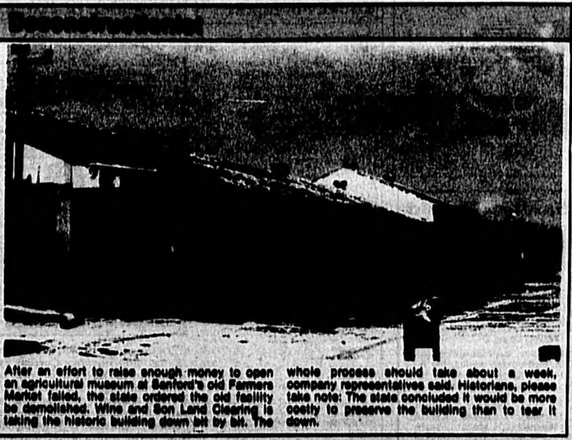
After an effort to raise enough money to open an agricultural museum at Sanford's old Farmers Market failed, the state ordered the old facility be demolished. Wine and Son Land Clearing is taking the historic building down bit by bit. The whole process should take about a week, company representatives said. Historians, please take note: The state concluded it would be more costly to preserve the building than to tear it down.
