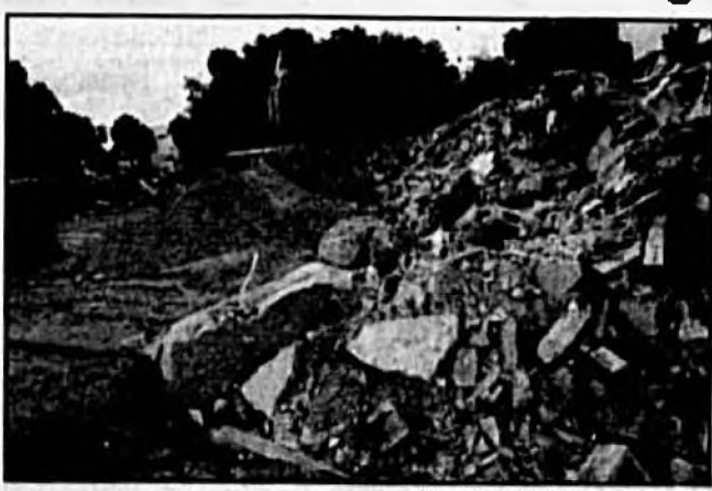
Demolish crews pile up debris from the old FP&L building next to Sanford City Hall. The property belongs to Seminole County.
