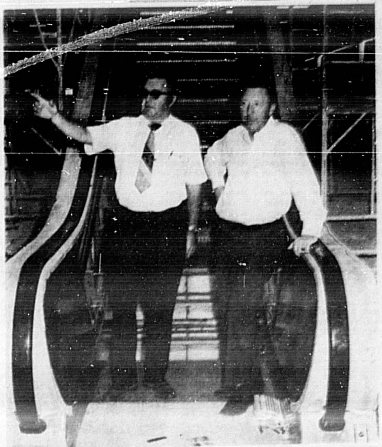
HAPPY ISON (left), Director of Public Relations, and Gordon Hulbert, General Manager, inspect construction progress at the Orlando-Seminole Jai-Alai Fronton. They feel confident that the construction will be completed and the fronton ready to open by October 2.
