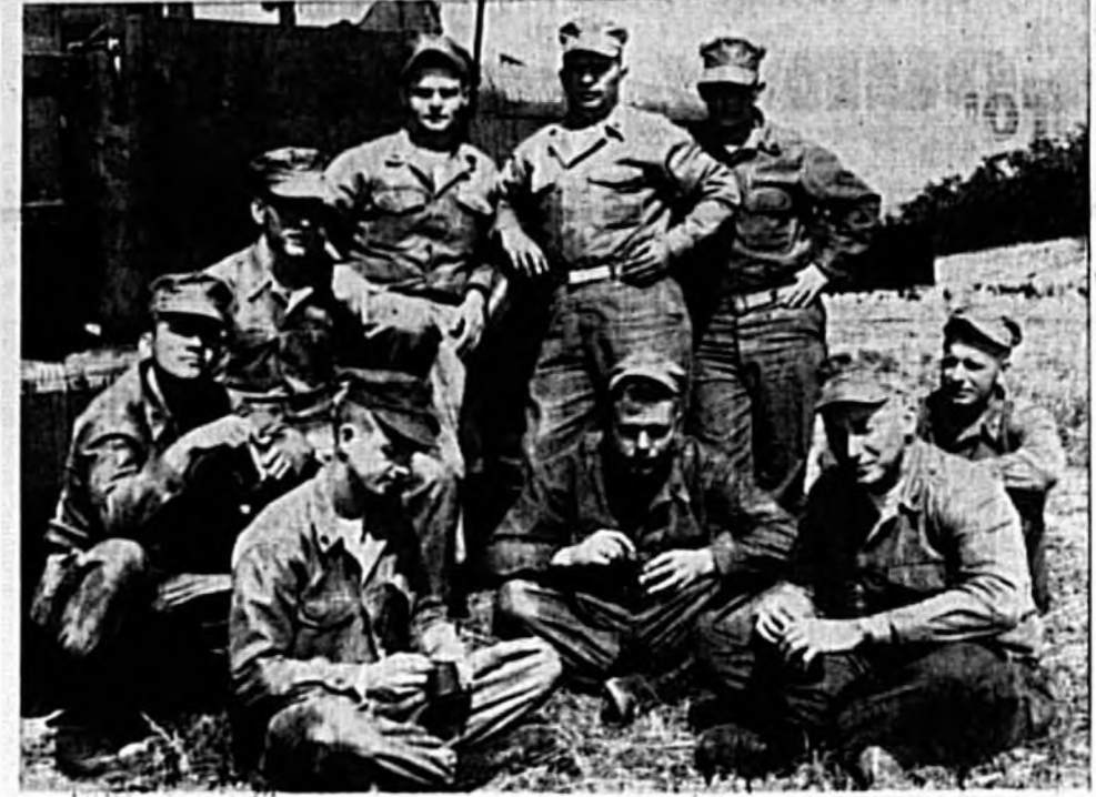
MARINE RESERVES from the Eighth Division Engineers break out C rations during lunch hour while clearing ground for the proposed Forest City Community Association Clubhouse. In the group are (seated, left to right) Cpl. W. R. Floyd, Cpl. J. M. Hunicutt, L. Cpl. J. E. Thompson, L. Cpl. A. P. Benson; (in back) Cpl. J. Garcia Jr., Cpl. R. A. Shuford, Cpl. M. J. Babb, Sgt. N. Fox and Sgt. W. H. Strickland. (Herald Photo)
