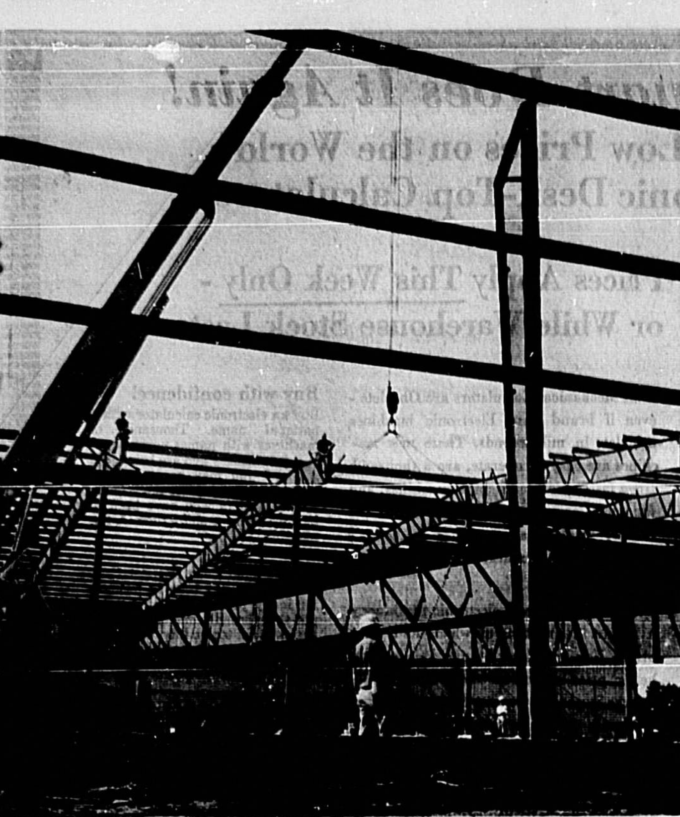
CONSTRUCTION IS proceeding on schedule for the new warehouse building of Port Everglades Steel Company (PESCO) at Port of Sanford. Here, a roof girder is being hoisted into place.
