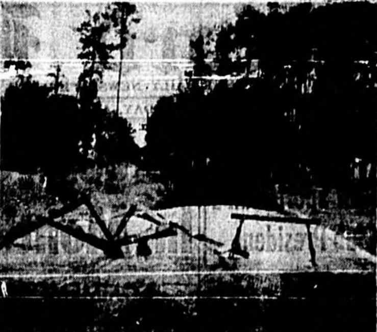
breaking rains. The hole develops when a line breaks and soaps down the sewer goes the surrounding sand. City Manager Tom Lemon (right) and Sidney Richard, superintendent of sewers (photo at far left) are shown at a cut-in on Locust Ave. between Second and Third Sts. Breaches in a 12-inch sewer caused this hole and other holes going on all day. Water stands in a
