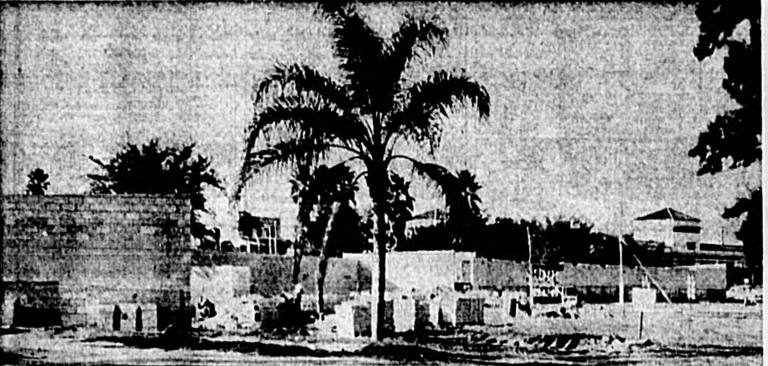
THE SANFORD CIVIC CENTER construction is on schedule and is expected to be completed by shortly after the year's end and ready for conventions and recreation programs.
