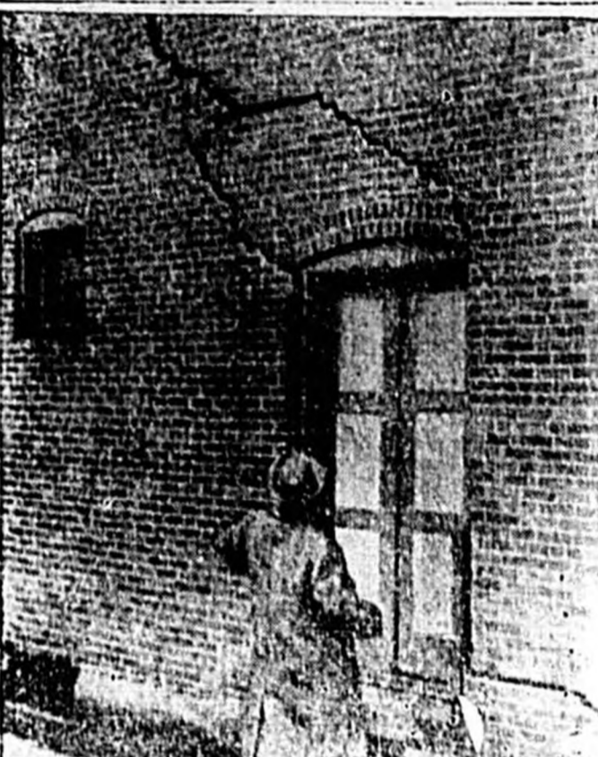
This picture, showing the crack in the wall of a mine town, was taken when a 100-foot wall of the town of Mineville, Pa., gave way last week. It is one of the many towns that have been abandoned because of the sinking of the earth.
