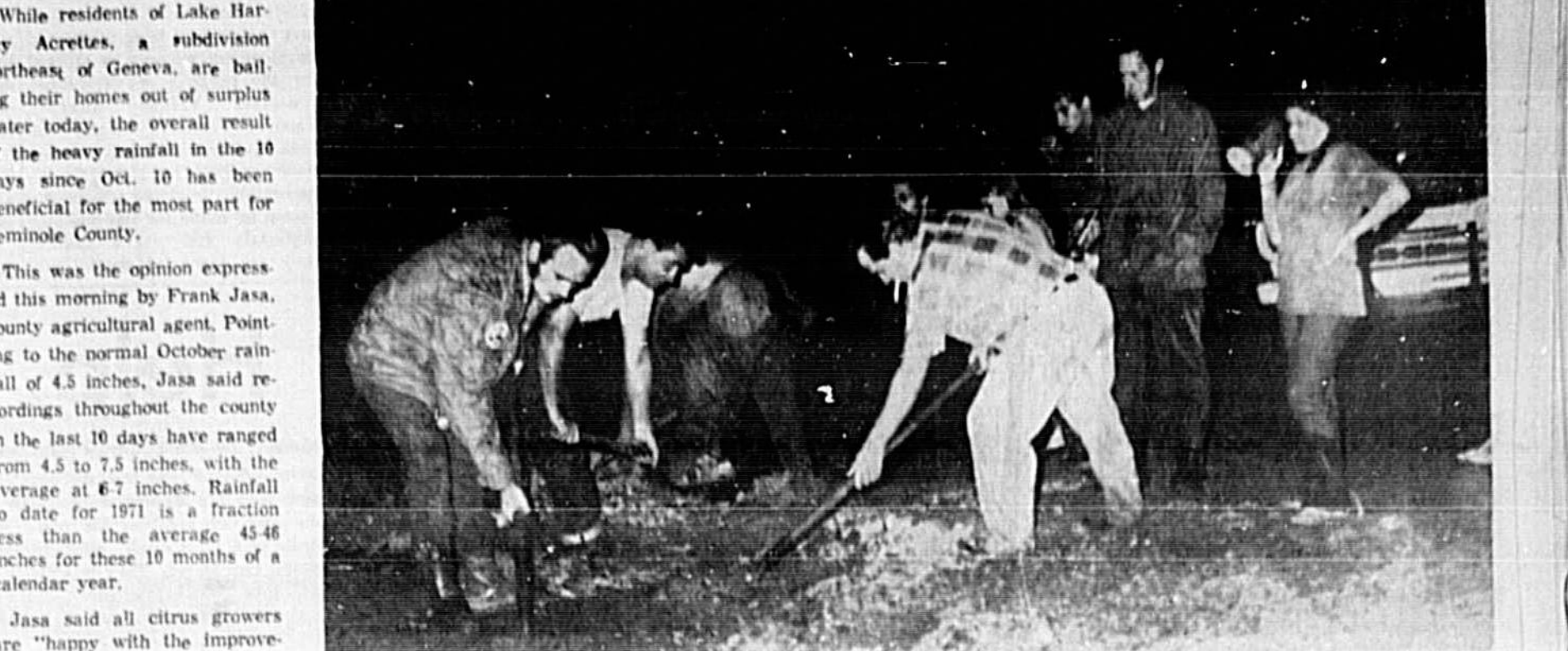
RAINS CAME... AND PROBLEMS, TOO Residents of the Geneva subdivision of Lake Harney Acrettes were out in the rain last night digging a ditch to drain their property. The group used cinder blocks and timbers to construct the ditch. One of the residents said he cannot get to his trailer with his car because the water is almost deep enough to use a boat. (Larry Neely Photo)
