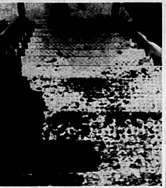
RUSTY STEPS — Up these rusty steps climbed 4,500 pairs of feet a year, children bound for a cooling swim. Now, with the pool off limits to the kids, the steps and the rest of the building still must be maintained, though not used, to protect the $50,000 investment.
