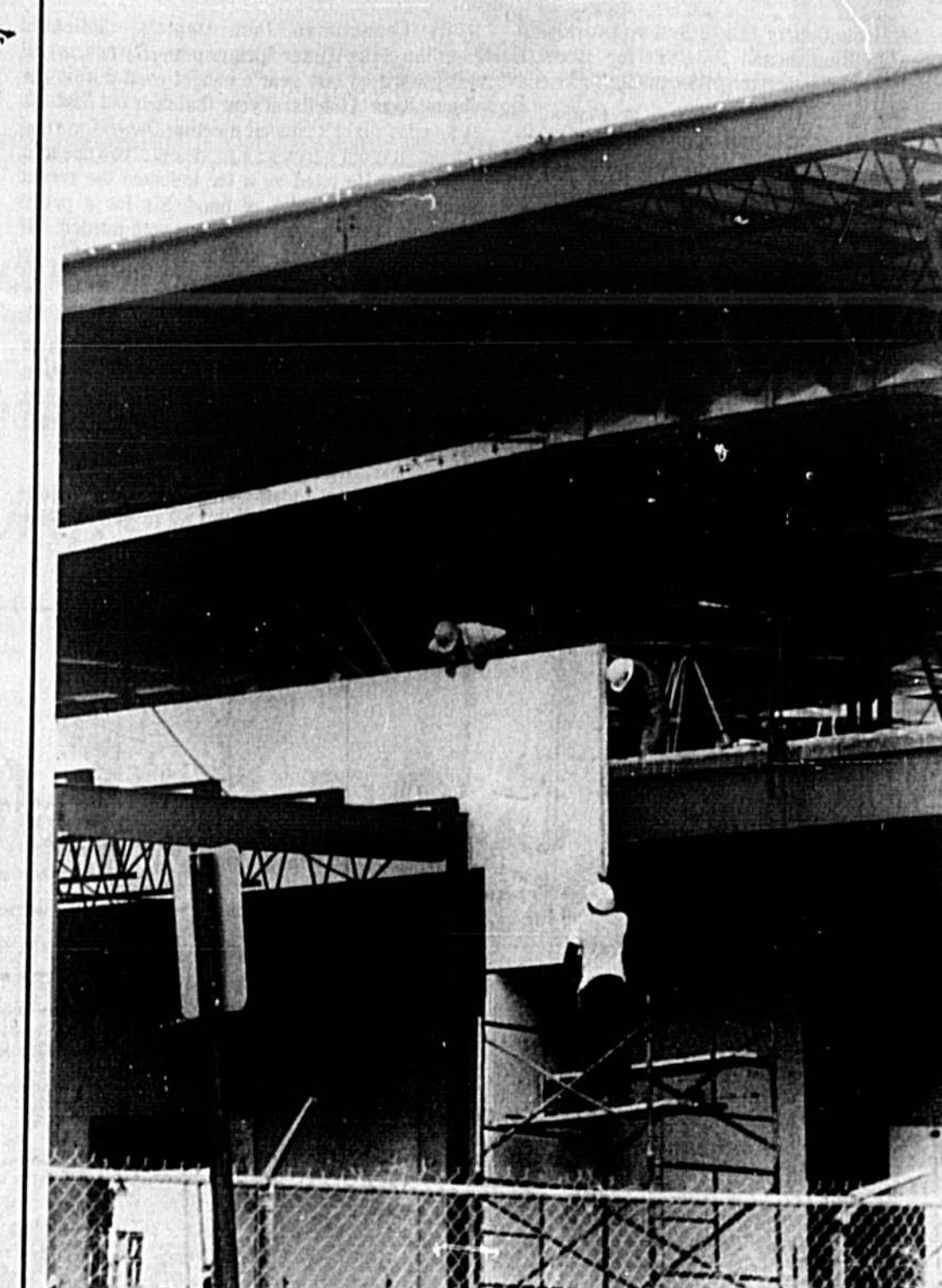
TARGET: DECEMBER Summer is about over and construction of the new $1.4 million Sanford City Hall is picking up speed — with a hoped-for completion in early December. The new hall will house offices for all department heads, except police and fire personnel.
