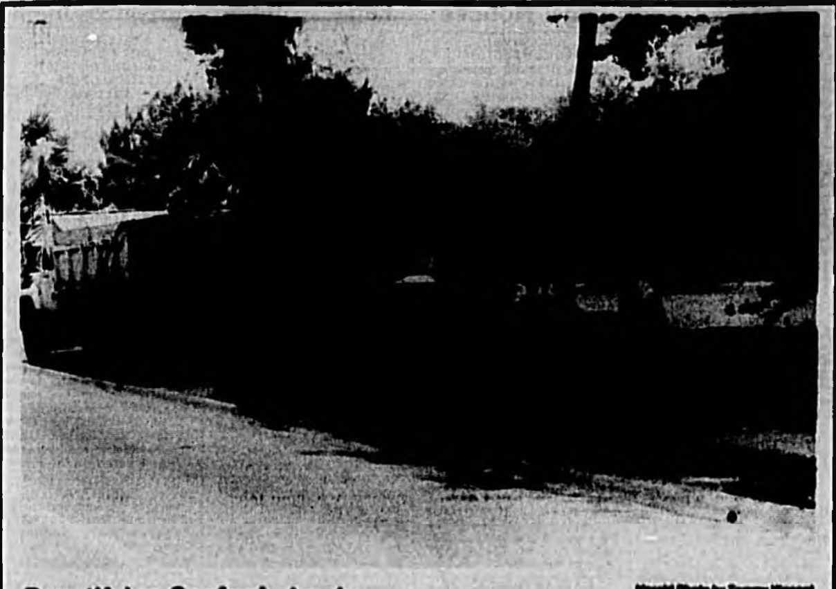
Beautifying Sanford streets Work continues along the edges of French Ave in Sanford from the lakefront to 25th Street. Cash, Clifford Watkins and Lynn Gooding, all Department of Transportation workers are now installing sod along the cleared area between the curb and sidewalk. Left to right, Freddie Cash, Clifford Watkins and Lynn Gooding, all Department of Transportation workers are now installing sod along the cleared area between 11th and 12th Streets.
