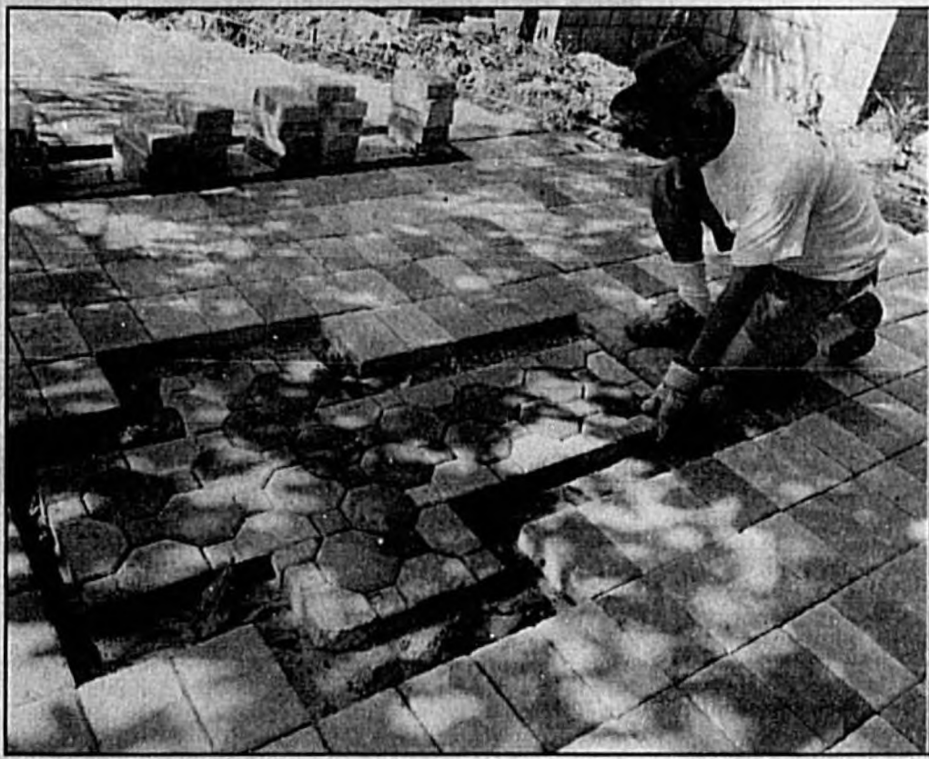
Herald photo by Tommy Vincent Tom West, founding member of St. Peter's Episcopal Church in Lake Mary, works on a section of a courtyard currently under construction at the church.
