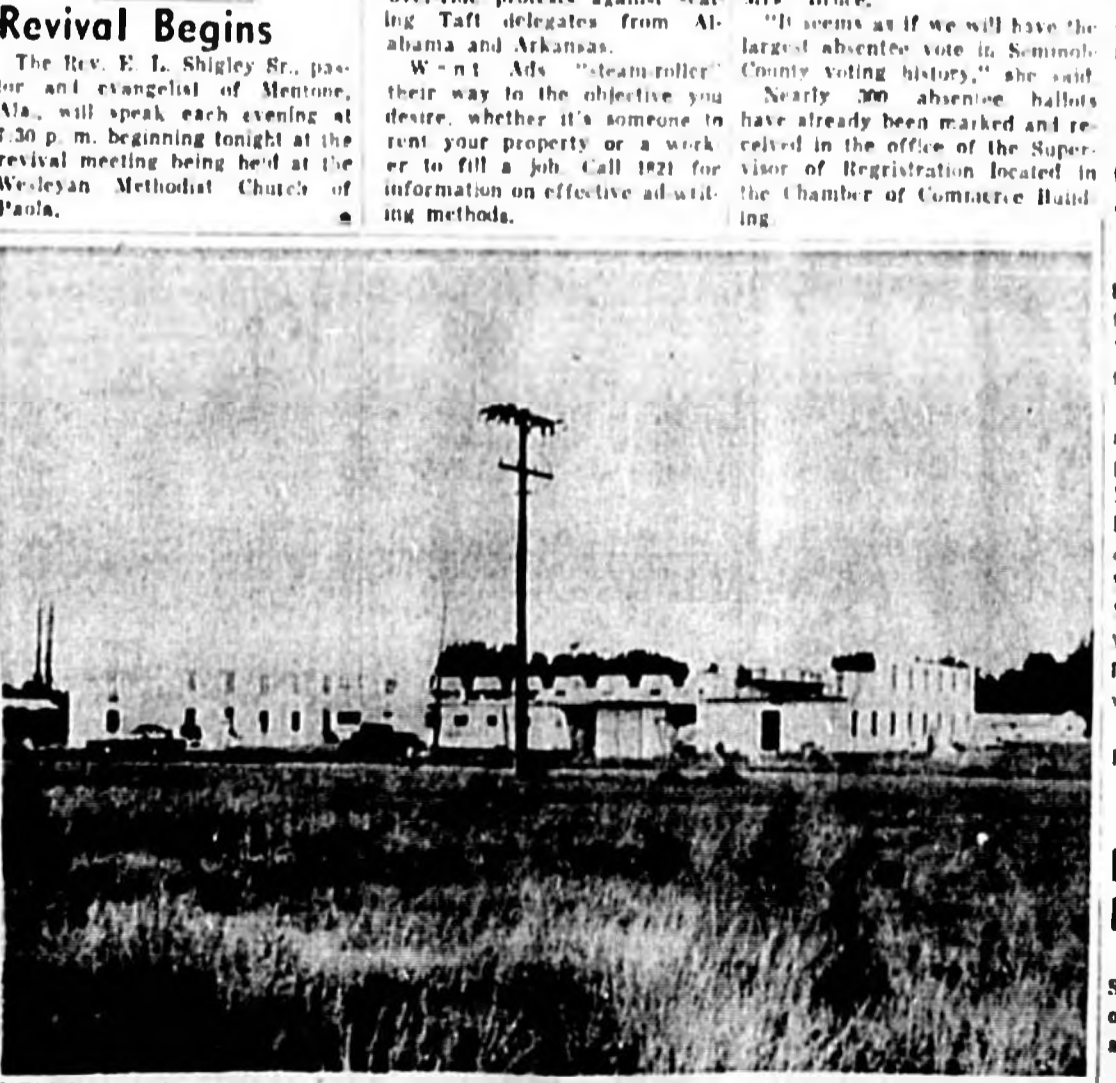
NEW YORK GIANTS dormitory building on Mellonville Ave. is about one-third complete. Date for completion of the sprawling building to house New York Giants Farm System is set for about mid-January. (Staff Photo)
