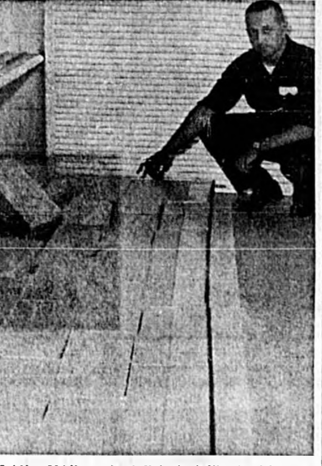
LAKE MARY School Principal Floyd Richards points to the school partition that fell Friday injuring three youngsters. (Herald Photo)
