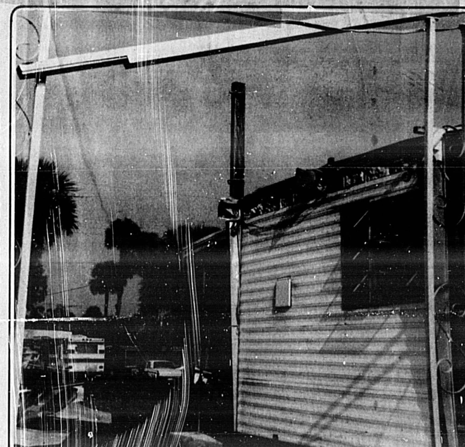
HIGH WINDS DAMAGE TRAILERS A sudden twister tore the roof off this mobile home (top) at Mullet Lake Park yesterday. High winds, rain and hail combined to damage mobile homes owned by W. T. Newton and Connie Sparks. The Newton 60-foot trailer was turned over on its side by the force of the wind. Debris was scattered throughout a wide area, such as wrapped around the utility pole at right, after the storm. (Herald Photos by Bill Vincent)
