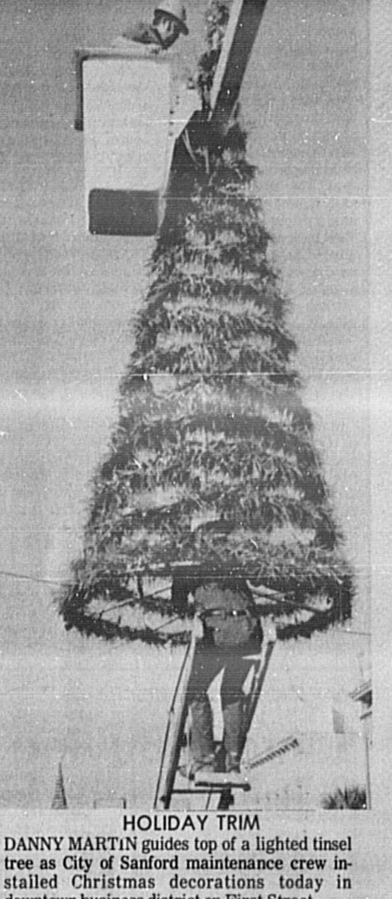
HOLIDAY TRIM. DANNY MARTIN guides top of a lighted tinsel tree as City of Sanford maintenance crew installed Christmas decorations today in downtown business district on First Street.
