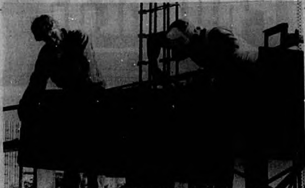
Mike Harrop, left, and Wayne Sperry connect a piece of wall beam on a new apartment complex off U.S. Highway 17-92 in Casselberry.
